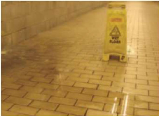
Wet slippery floor
